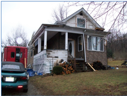
After the 2006 Fire Workers have torn off the old aluminum siding and are getting ready for new vinyl siding. The inside has been totally gutted and remodeled.
